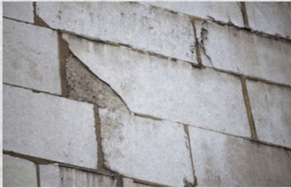
Rusting cramps damaging ashlar face
