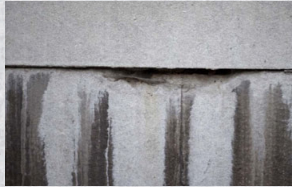
Rusting cramps damaging ashlar face
