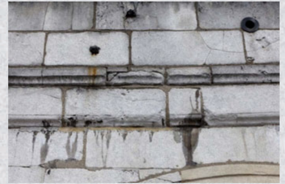
Staining and parapet cracks
