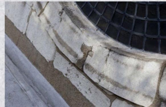
Cement mortar fillet; ferrous cramp damage
