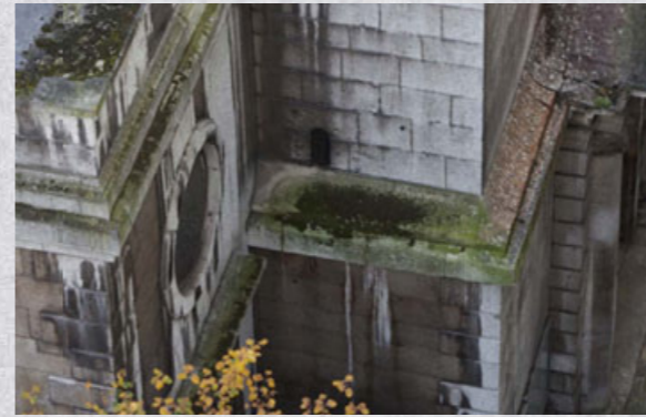
Heavy staining and bird pollution
