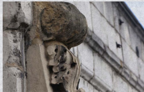
Parapet cracks; sculpture erosion; inappropriate pointing
