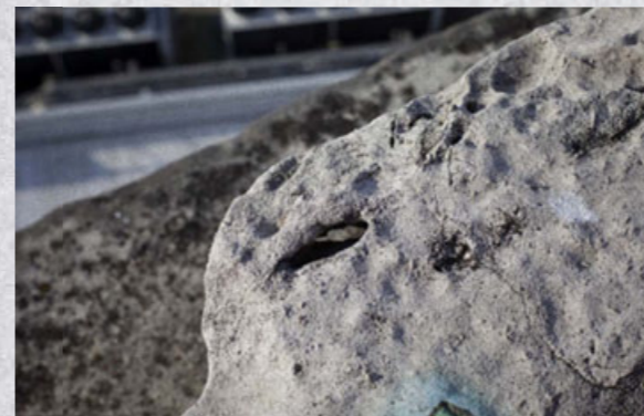
Heavy erosion forming hole in cornice
